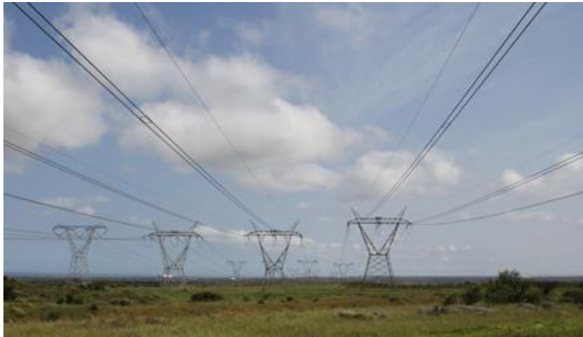
Figure 43 Eskom high voltage power lines south of Atlantis SEZ
