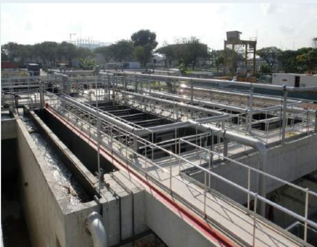
The UASB-Ceramic MBR plant
