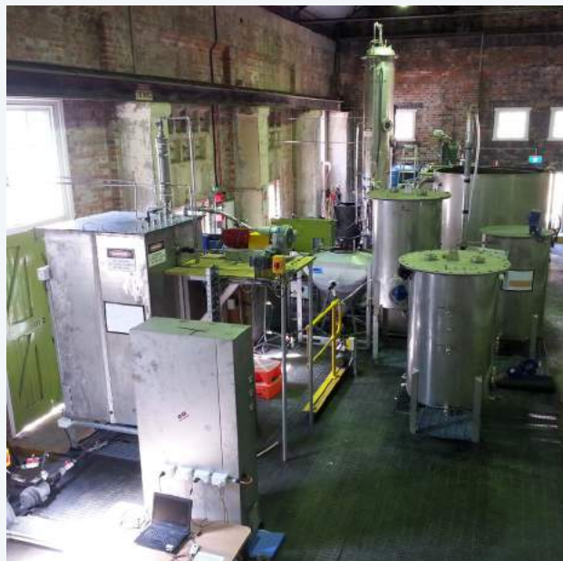
The Anammox pilot plant trial at Queensland Urban Utilities (QUU) wastewater treatment facility at Luggage Point, funded by AWRCE
