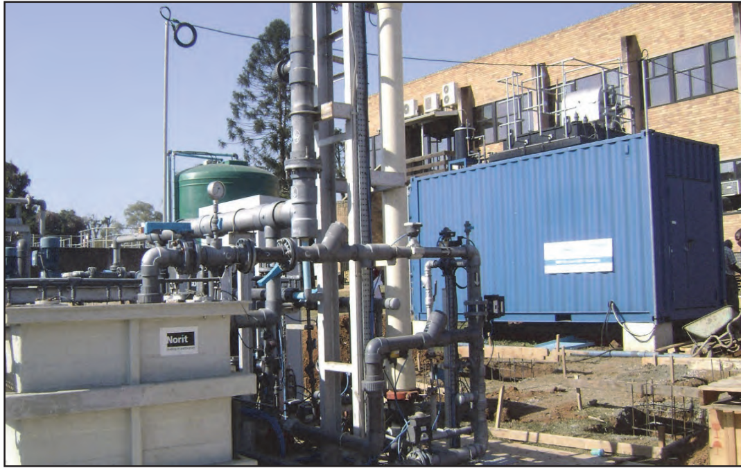
Figure 3.4: Norit MBR Pilot Plant Showing External Membrane Module
