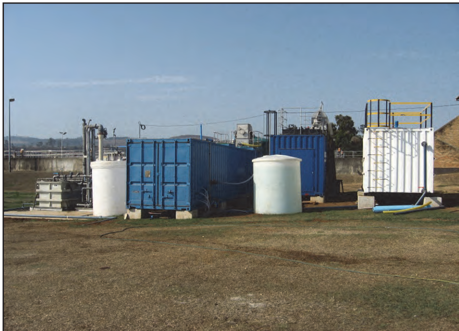
Figure 3.2: Onsite MBR Pilot Plant Set-up
