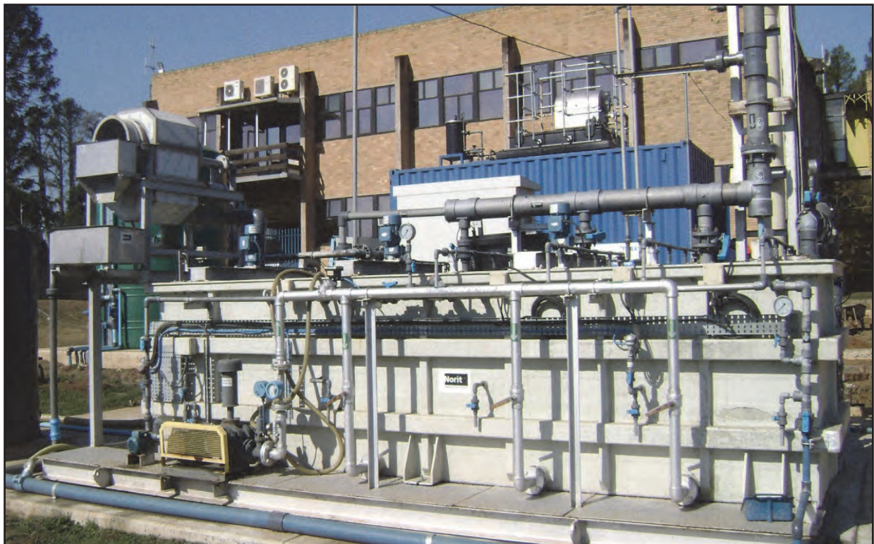
Figure 3.3: Norit MBR Pilot Plant showing Drum Screen
