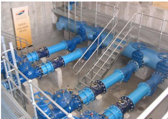
Fig 2: Pressure Management Chamber in Cape Town (source, Meyer et al, 2009)
