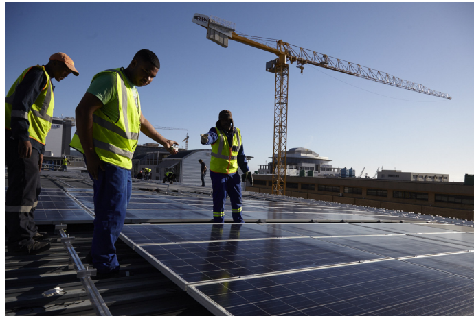
Rooftop solar photovoltaic panels being installed by SolaFuture on the Takealot.com building in the Cape Town central business district. The system will generate 780,000 kWh per annum, enough energy to power 100 medium sized houses.
