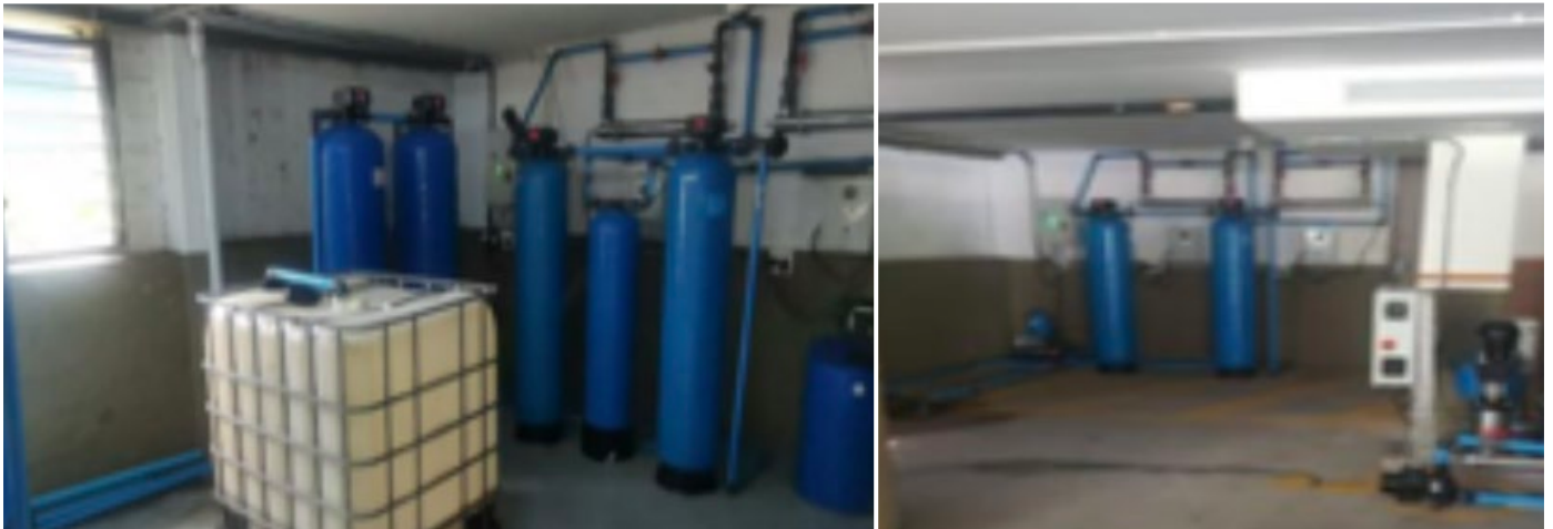
Figure 2: The water filtration plant installed at the Southern Sun hotel in Newlands
