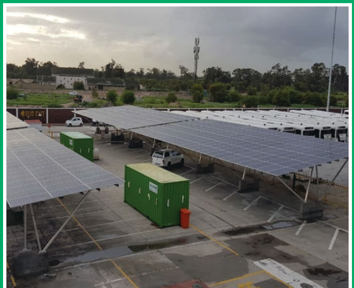
Figure 4: Solar PV Car Port at the GABS depot near the Cape Town International Airport (Source: GABS, 2022)
