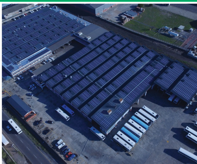
Figure 3: Solar PV rooftop installation at the GABS head office in Epping, Cape Town (Source: GABS)
