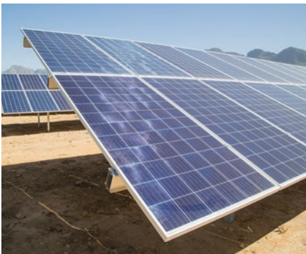
Ground mounted solar PV
