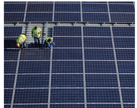
Rooftop solar PV
